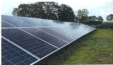
Great Bay Solar Project (118 MW) Westover, Maryland
